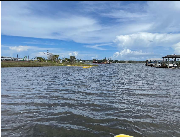
Photo 4: Typical view of turbidity barrier and manatee signs as well as 20' Wide Barge being pushed back to Baseline 2.
