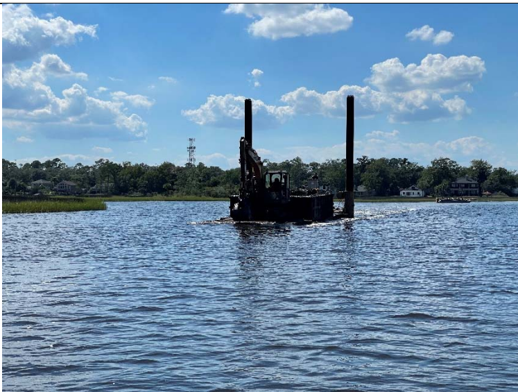
Photo 2: View of 26' Thruster Barge heading to off-load. Barge currently dredging in Baseline 1: South IOP
